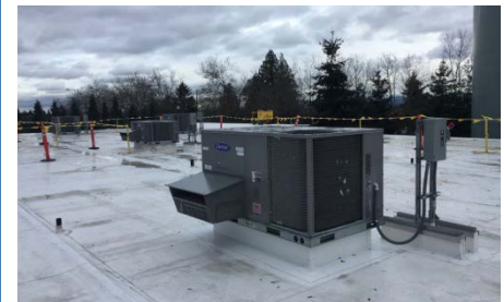
Water Tower Field Office HVAC Unit
